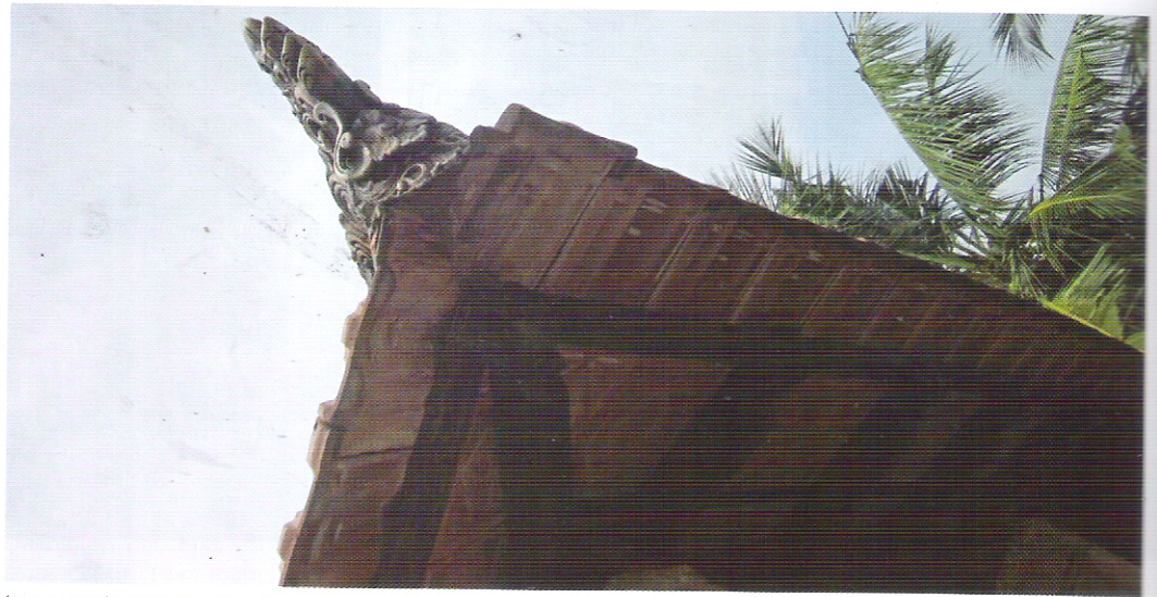
interpretation of the Drip Edge through Balinese edge tiles; Residence on the beach, Chennai.
