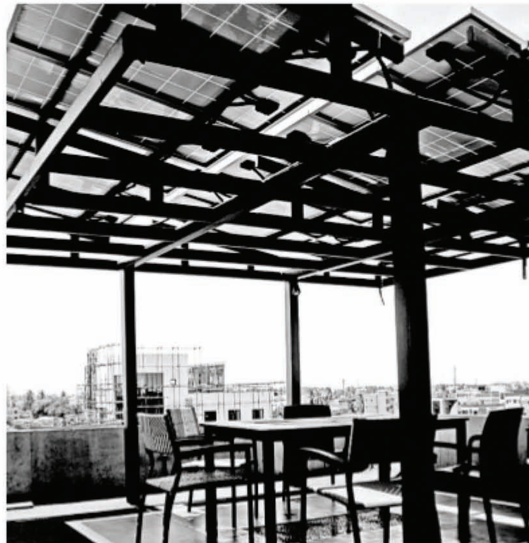
A rooftop photovoltaic system offering both shade and electricity • Express
